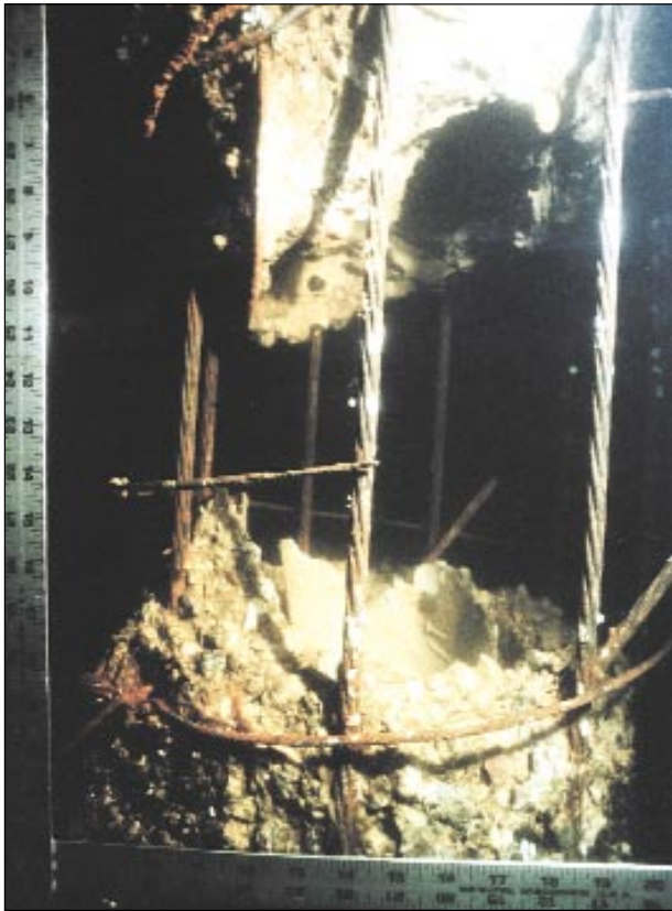
Left: Chemical reactions, such as sulfate attack, DEF, or ASR, can cause extensive damage. Below: An important consideration with breakage defects is restoring the load to the member after it's been repaired.
