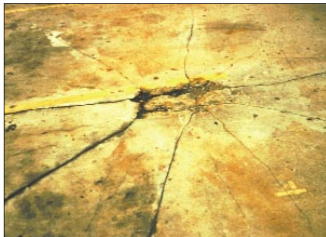
Cracks radiating from a supporting column are a structural failure indicating that the slab is overloaded.
