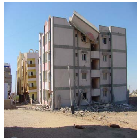
Fig.10 5 storey R.C., collapse of open plinth, water tank at top dislocated (Bhuj)
