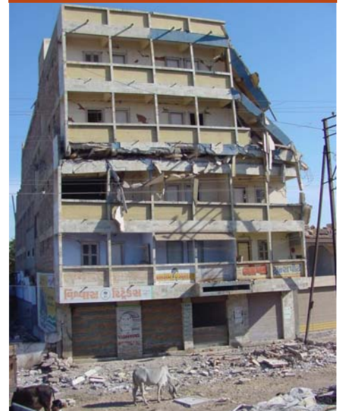
Fig.8:- Collapse of soft middle storey in a building at Bhuj.
