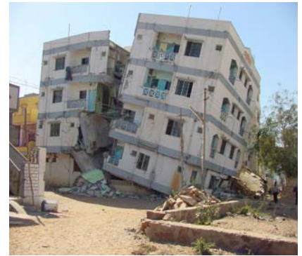
Fig. 6 Soft Storey (Open Plinth), Vertical Split between two blocks (Bhuj)
