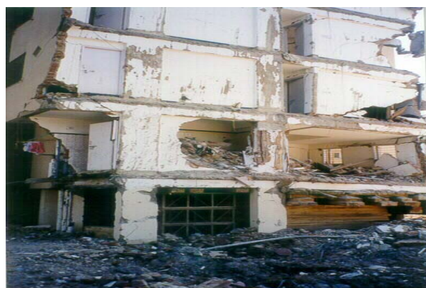
Fig. 17:- Infill wall damage
