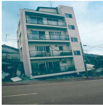
Fig. 5 Soft first storey collapsed, upper part of the building fall onto the ground, (kachchh, 2001)
