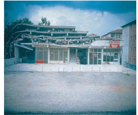
All the upper floors weak in long directions (Izmit, Turkey 1999)
